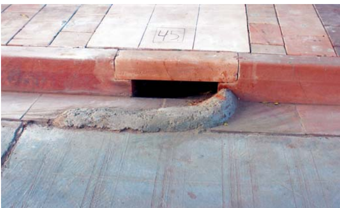
Inlet for road side drainage
