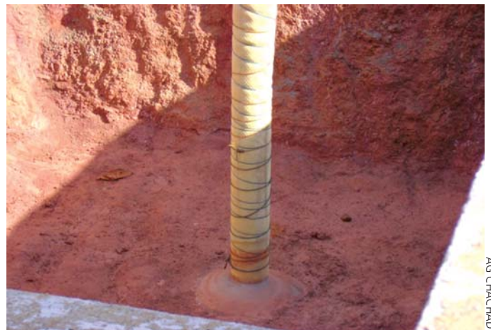
Deep recharge bore well
