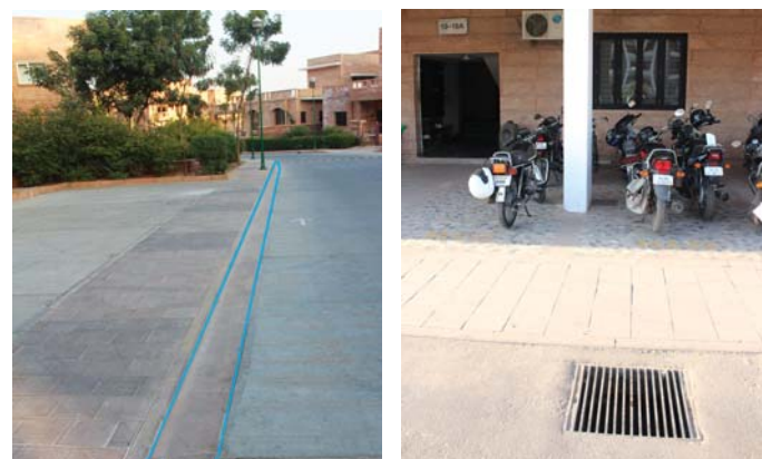
Open channels and grated underground storm water drains
