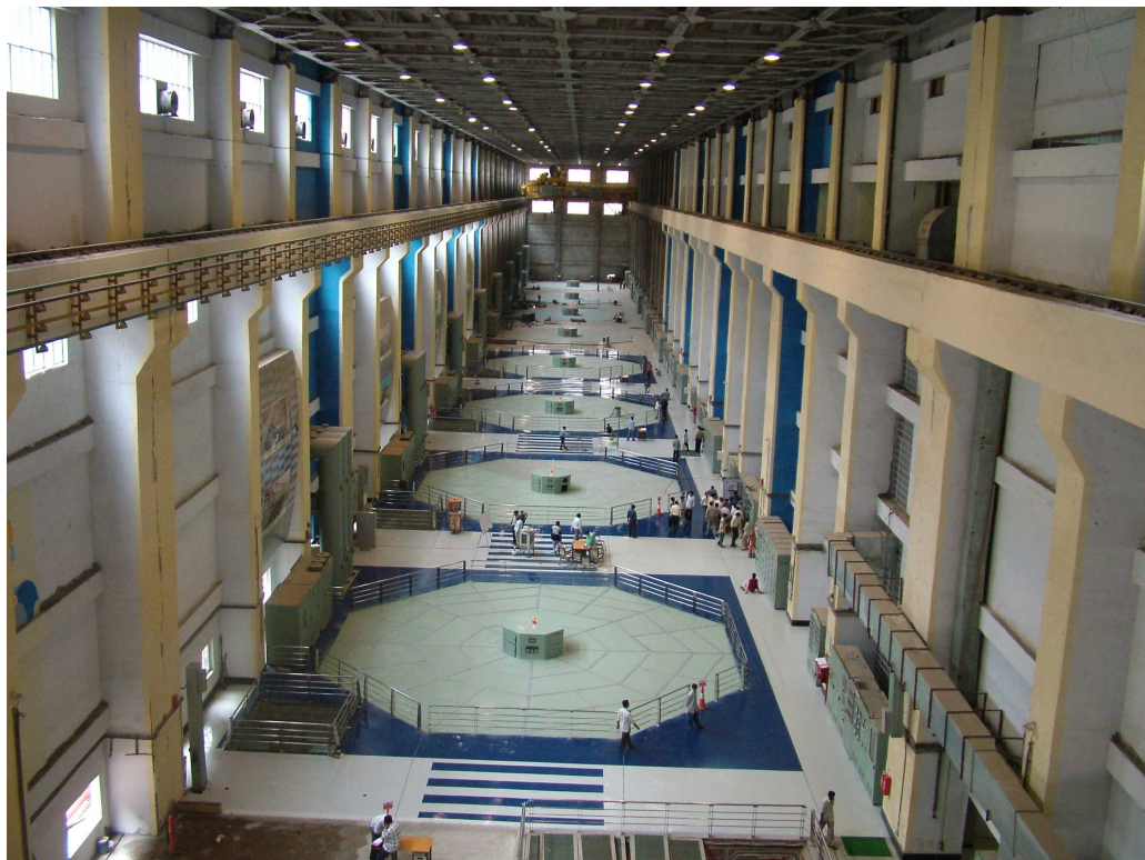
Machine Hall of 1000 MW Indira Sagar Project
