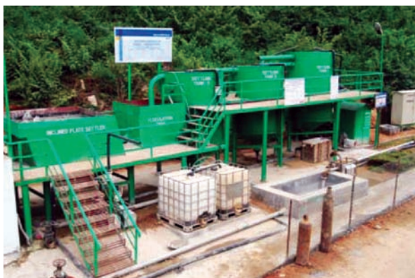
Water Reuse Plant at HCC's Vizag Cavern Project, Andhra Pradesh
