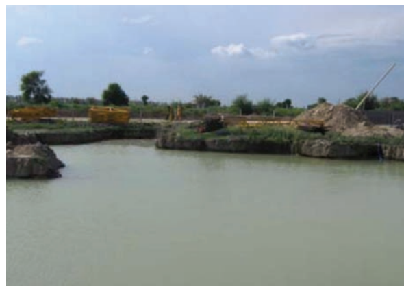
Mirzapur Artificial RWH Pond at HCC's Badarpur Elevated Highway Project, Delhi
