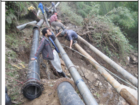
Plate 3: Water supply pipes broken due to heavy rains in Ratey Chu (2 nd week of April, 2007) (Source: C.D. Bhutia)
