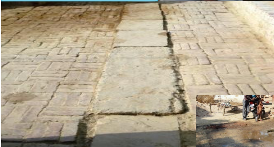
Central drainage system for secure village health
