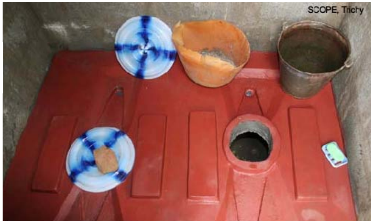
Drop hole in the middle, urine hole with proper slope in the front wash water bowl in the rear
