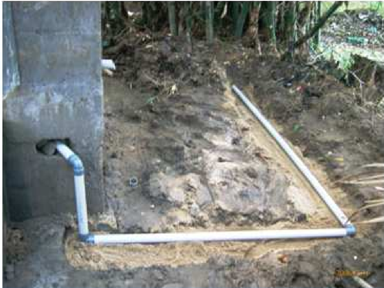
Pipeline for urine & wash water
