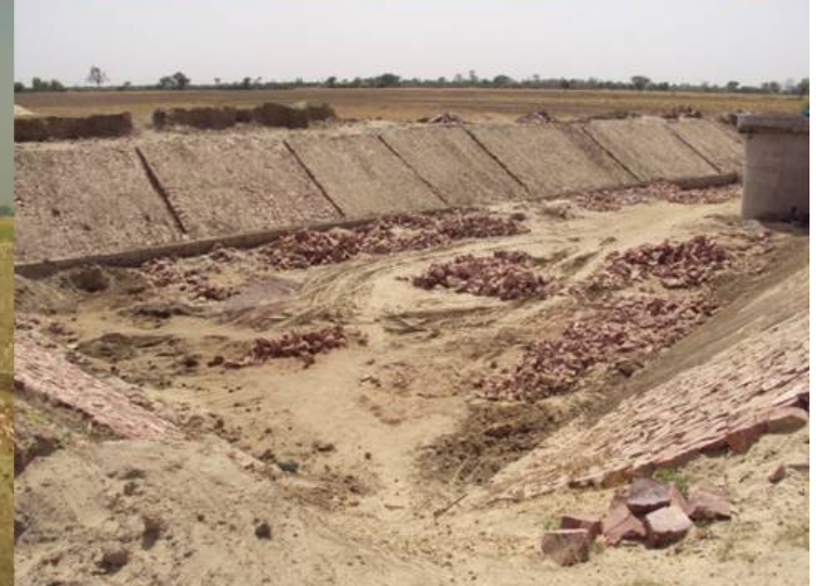
Settling of the soil
