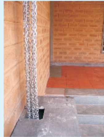
Chains leading the roof water to the filter
