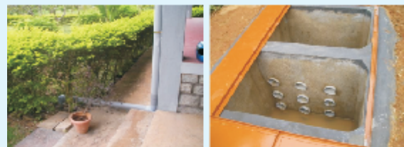
PVC down-take pipe
