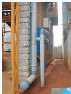
The first rain separator with an end cap used as a by-pass when cleaning the roof
