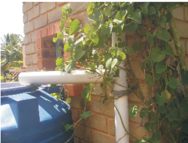
Elbow Junction & Tee Junction
