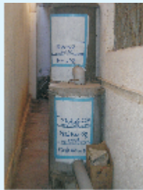
The filter and sump tank
