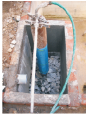
Recharge pit around bore-well
