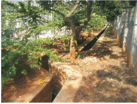
Open drains collecting the rainwater
