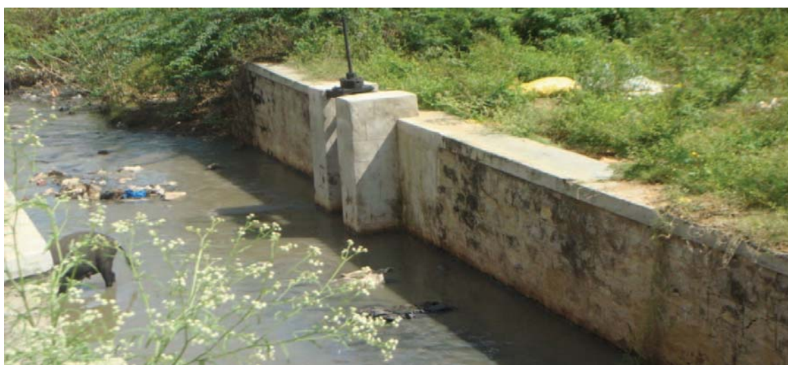
Blocked I&O at Davanagere
