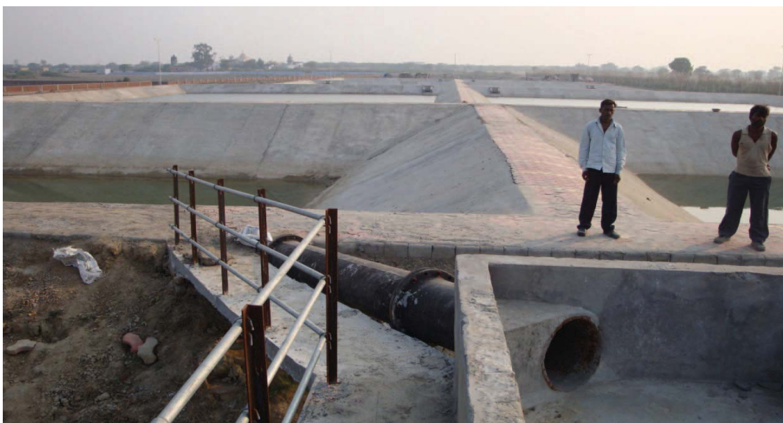
Incomplete STP 2.76 mld (WSP technique) at Mathura
