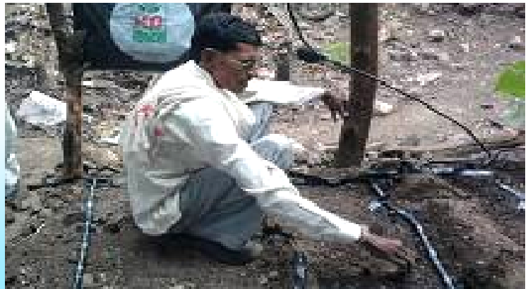
Drip pipes with sac laid in kitchen garden developed by the More family
