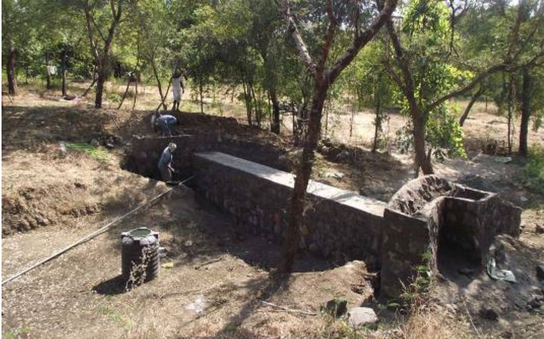
Construction of Nala Bund/Check Dam at Rajbhavan at Nagpur under CSS of ARP
