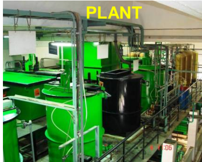
EFFLUENT TREATMENT PLANT
