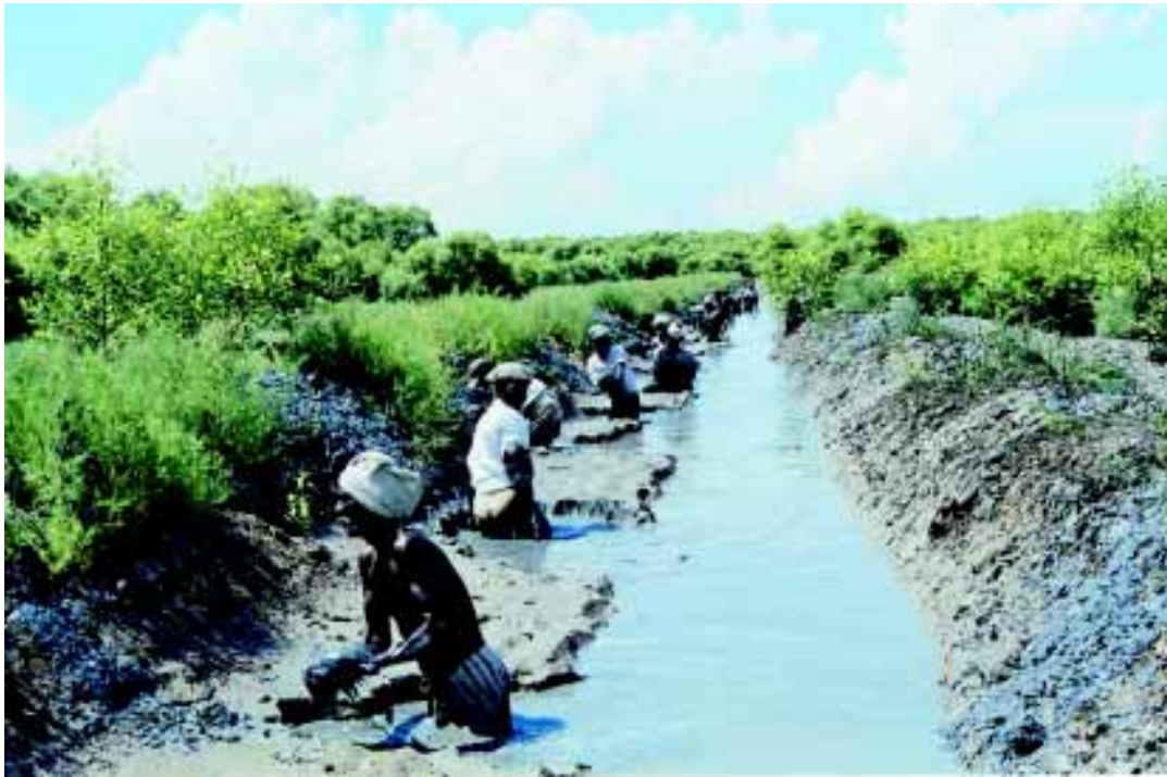
Figure 3.15 a. Desilting of the canals is one of the important tasks of mangrove management
