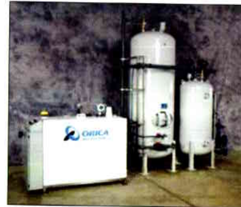
Figure 6.4: MIEX® Treatment Systems
