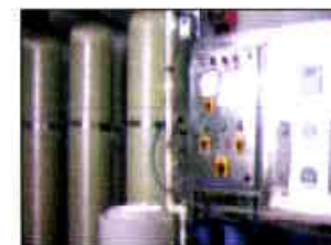
Figure 3.14: RO technology, IICT, Hyderabad
