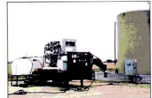
Figure 7.6: A&M mobile desalination unit
