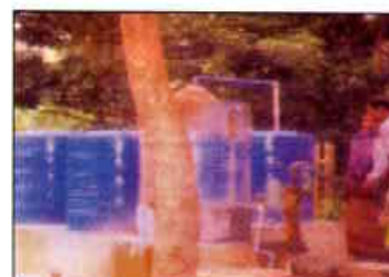
ARSENIC TREATMENT PLANT- PHED MODEL
