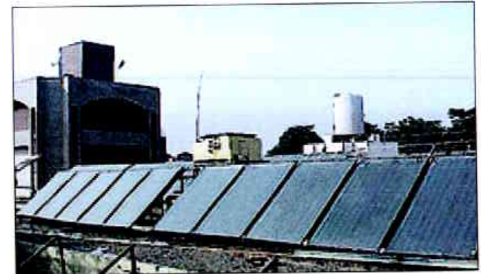
Figure 7.3: Flat-plate-collector-based solar desalination system installed at the Solar Energy Centre, Gual Pahari, Gurgaon
