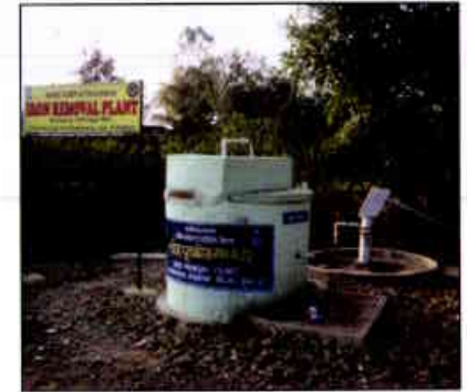
Figure 5.1: NEERI hand pump attachable iron removal plant
