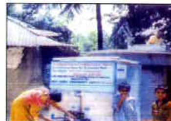
HANDPUMP ATTACHED ARSENIC REMOVAL PLANT-AIHH & PH
