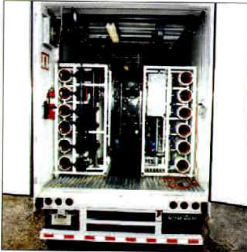
Figure 7.2: Siemens Water Technologies
