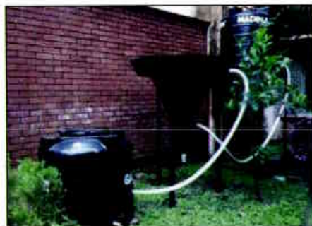
Figure 4.32 : ARUBA Arsenic Removal Plant Prototype
