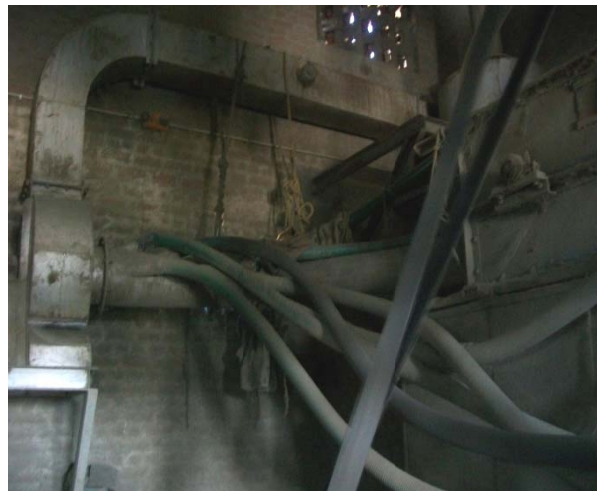
Fig 5.20-Variou suction ducts from milling section to a common cyclone in small rice mills
