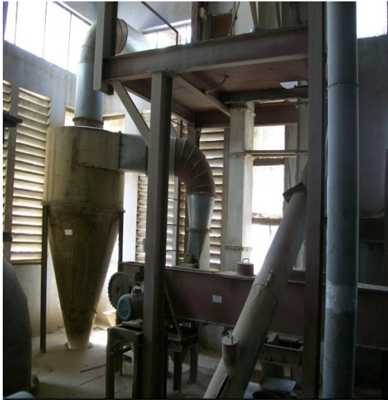
Fig. 4.4- Dust extracted through Cyclone
