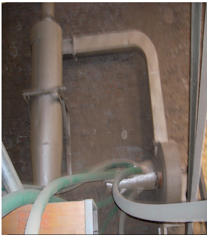
Existing Dust Extraction cum Control System
