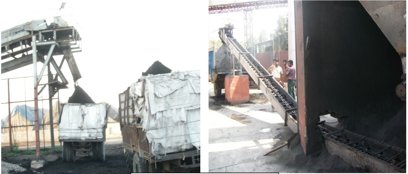
Fig 4.13-Mechanical handling of boiler ash
