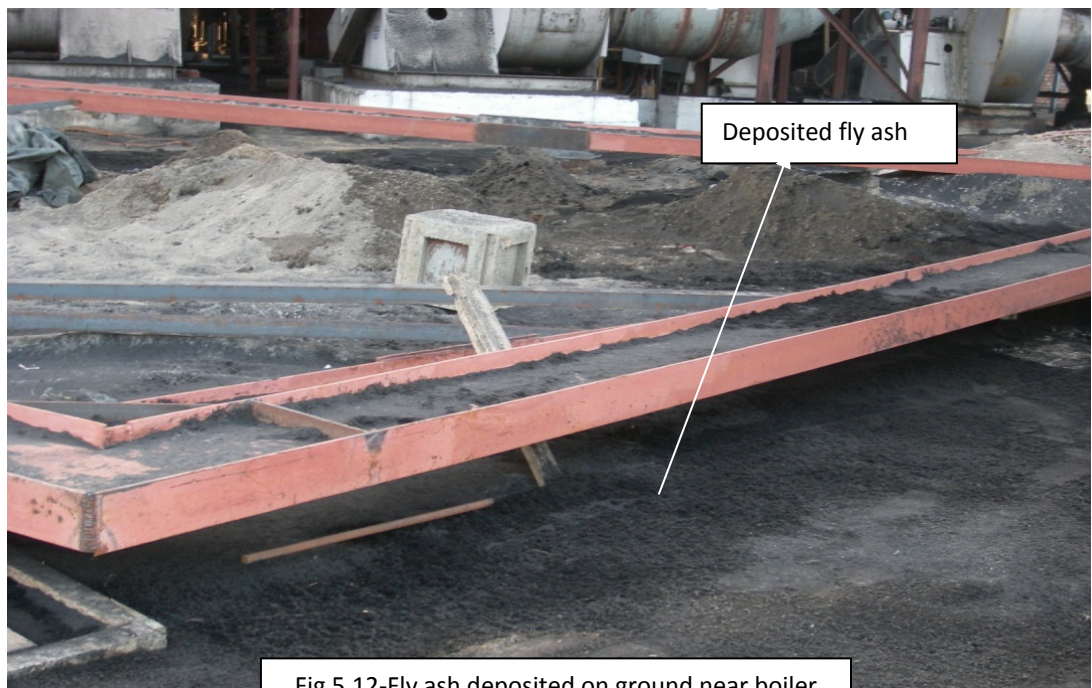
Fig 5.12-Fly ash deposited on ground near boiler section due to Fugitive Emissions
