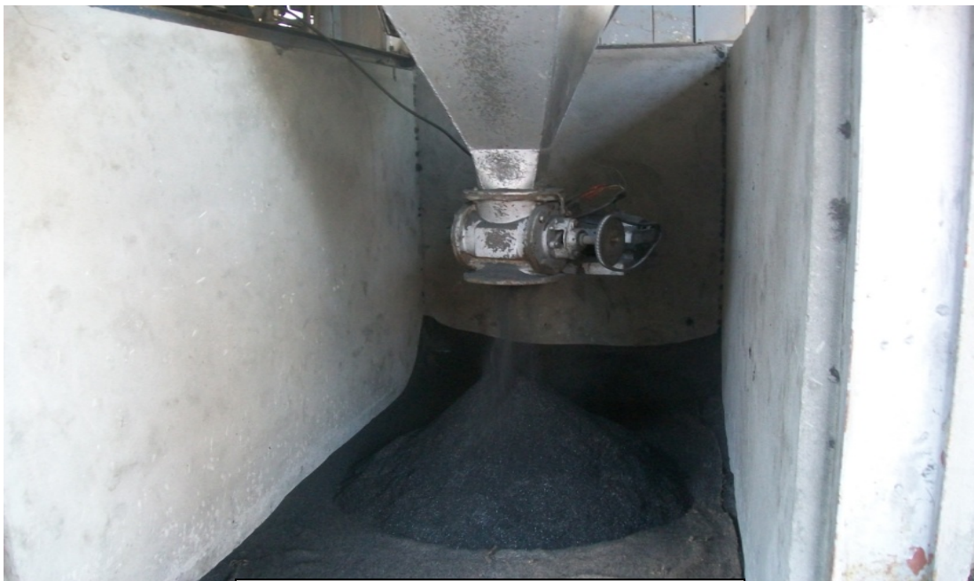
Fig 5.22- Cyclone for collection of boiler ash in large and medium rice mills
