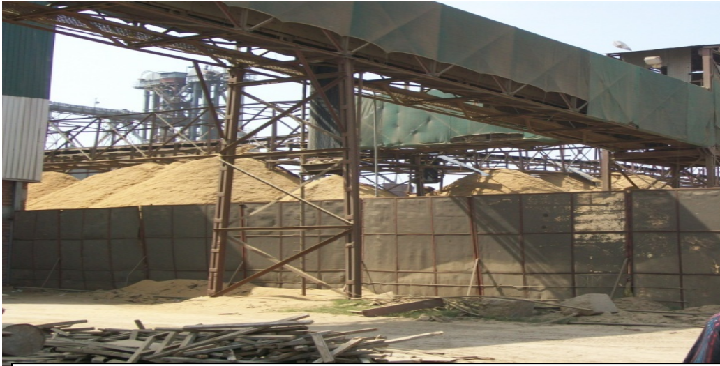
Fig 4.11-Husk Handling from storage yard to boiler using conveyor belts in large mills
