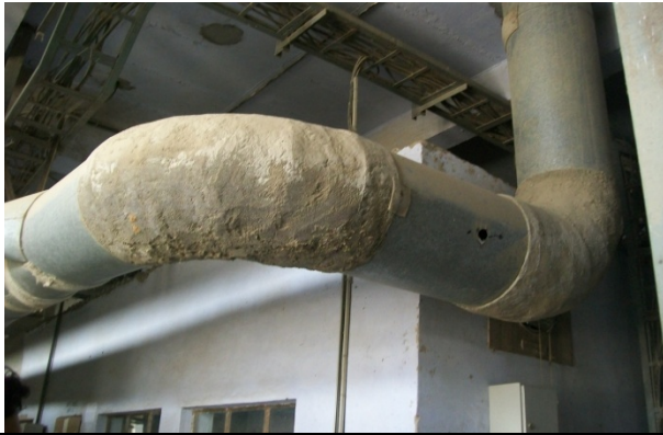
Fig.6.7. Common Duct from Paddy Separators (2 nd floor)
