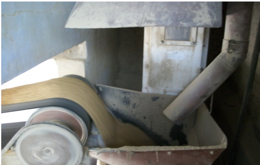
Fig 5.16-Extraction Hood near Bucket Elevator in large mills
