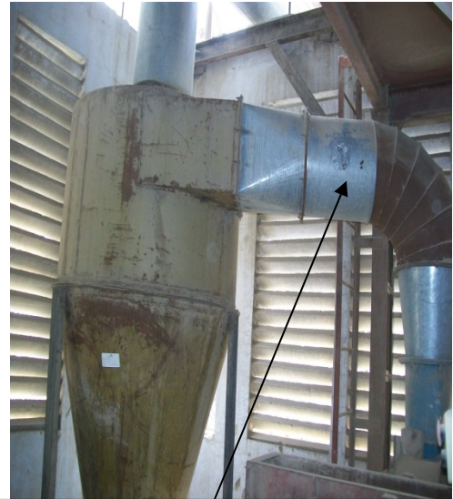
Fig.6.10. Cyclone Inlet (Port Hole 7) on 4 th floor
