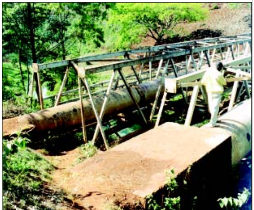
Plate 10. Nairobi City water supply pipes from the Nkaini reservoir.
