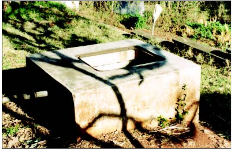
Plate 3. A vandalised inspection covers for a sewer drain. Stones and other objects may fall in and block the drain.
