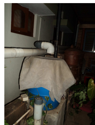
You can clearly see the material used to filter the rainwater
