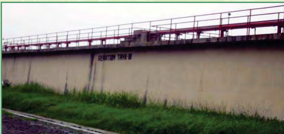
Defunct aerator tank
