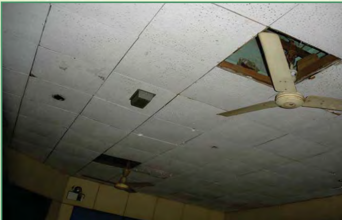
Poor condition of galleries
