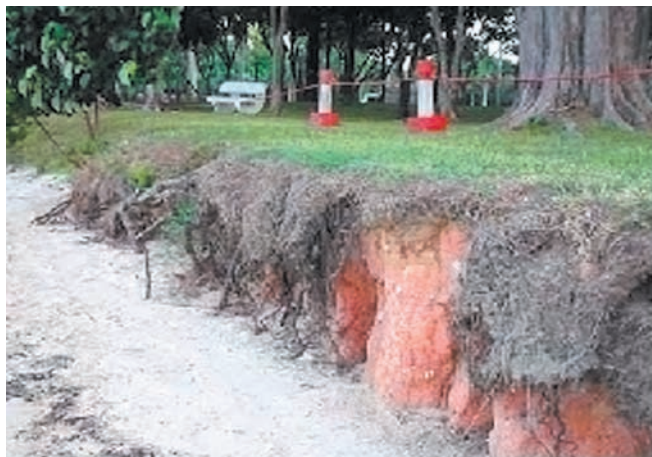
Figure 3.10. Coastal Erosion at East Coast Park, Singapore
