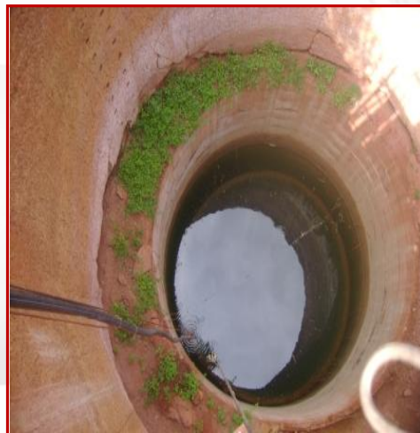
Open well under usage
