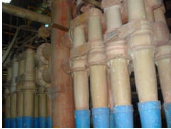
Picture before modification Water requirement : 6m 3 /hr
