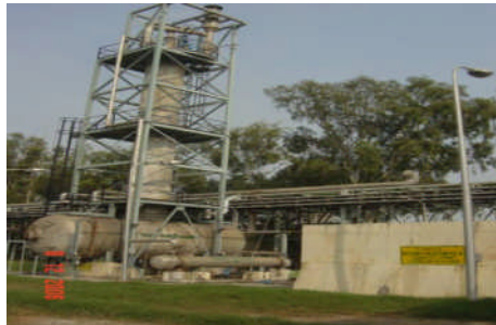
Effluent Treatment Plant Cost : Rs. 203 Lakh
