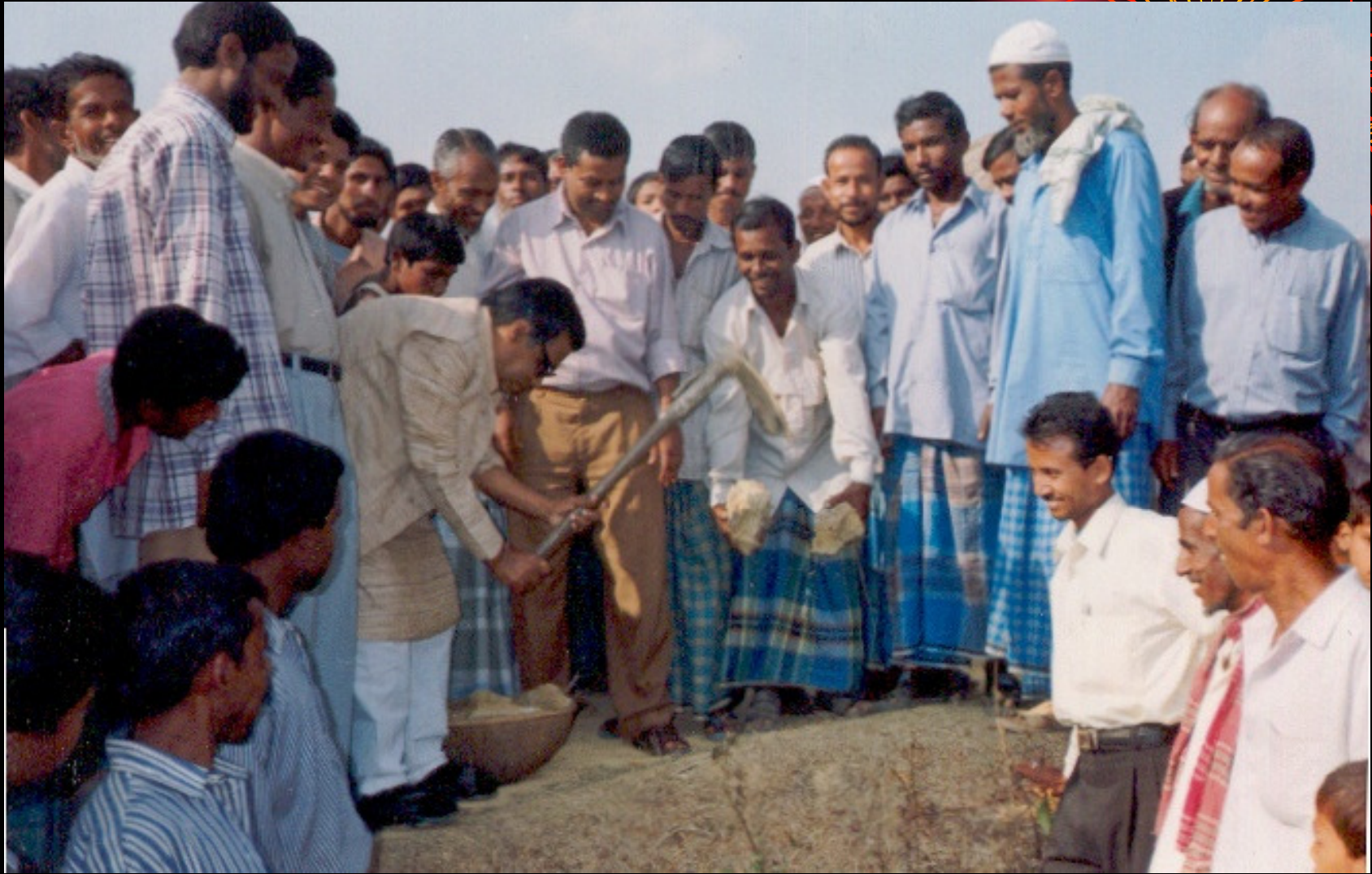
Constructin of Tulakuna Road inaugurated by Late Madhabendra Dutta Choudhury under Entry Point Activity
