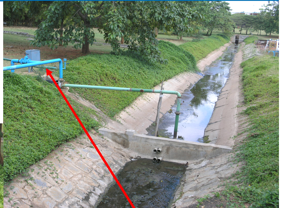
Pump installed at Open canal
