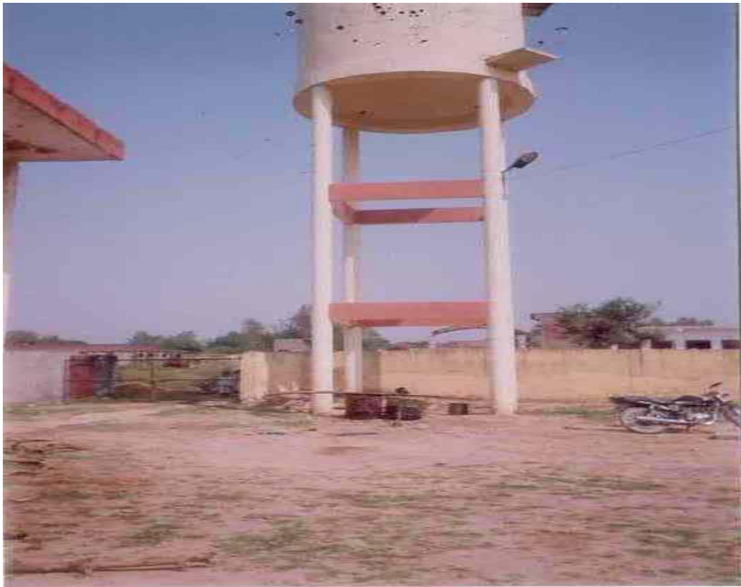
View of Single OHT of 50 KL at VWSC Dalpatpur, Moradabad District
