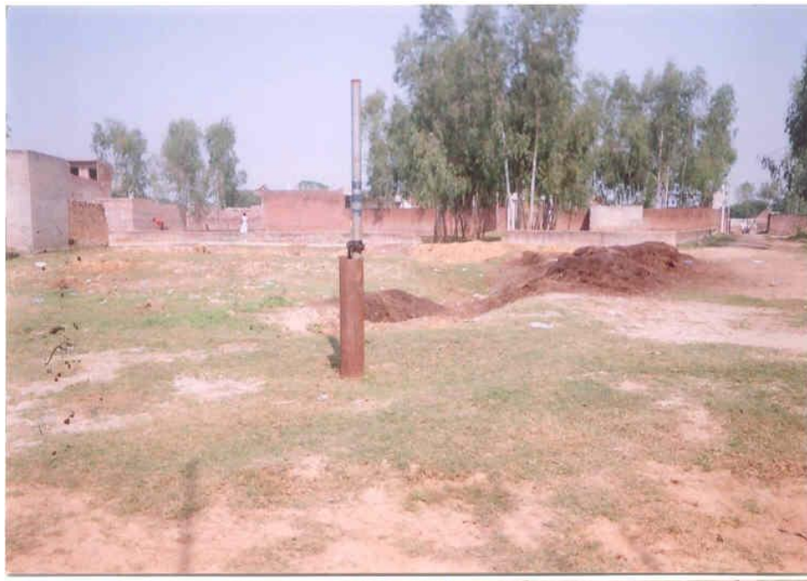
Incomplete Pumphouse at VWSC Sarkara Khas, Moradabad District
