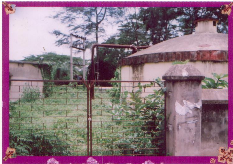
Underground sump for Bishwanathpur PWS in Puri District constructed prior to 2003, reported as commissioned in 2005, remained uncommissioned.
