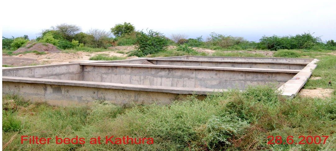
View of WSS, Kathura lying incomplete
