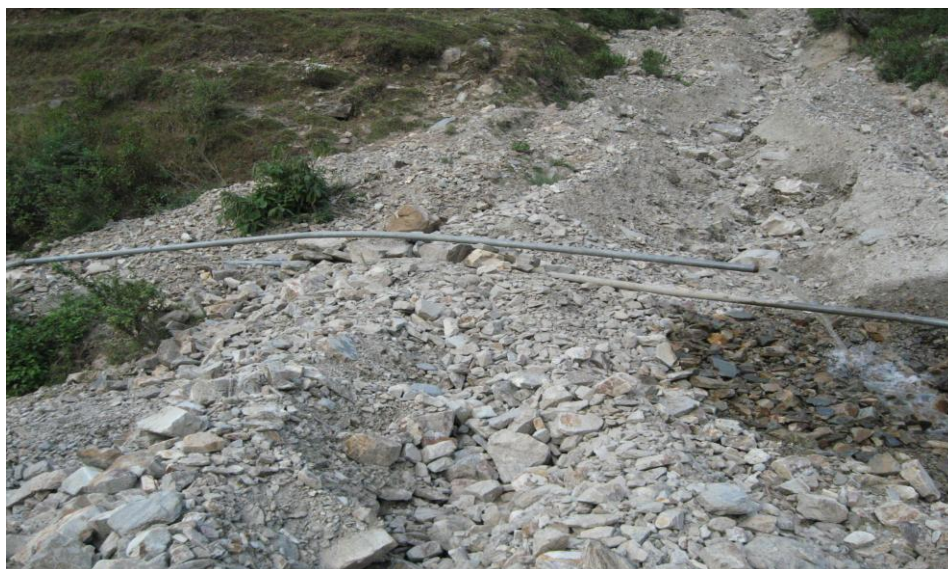
Broken intake pipeline for Bunga Jawari WSS, covering four habitations and two primary schools
