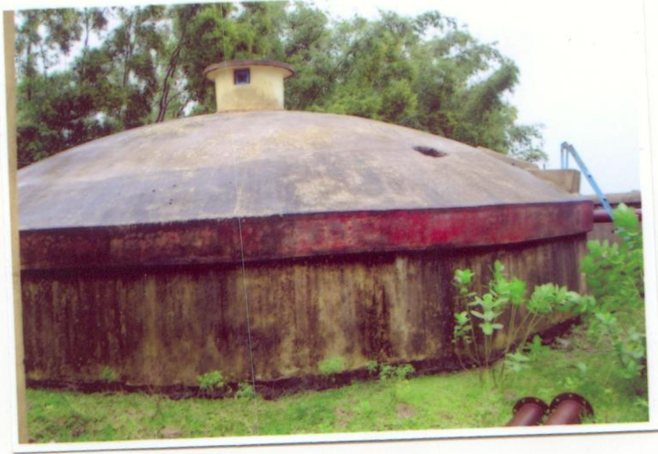
Underground Sump of Bishnupur RPWS constructed prior to 2003, which remained uncommissioned
