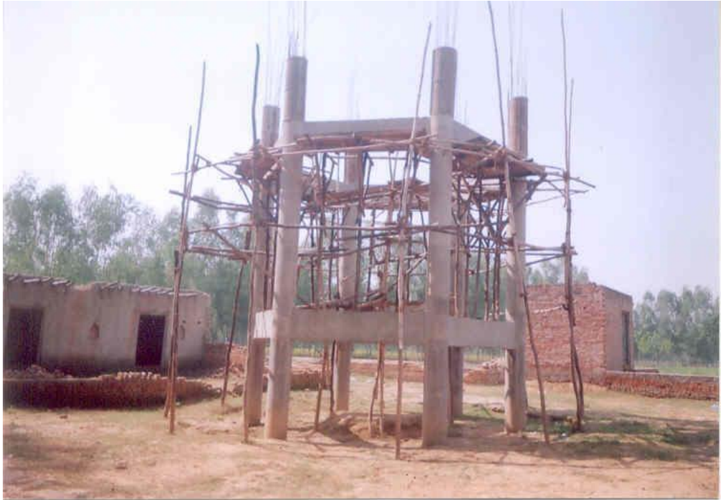
Incomplete OHT at VWSC Sarkara Khas, Moradabad District
