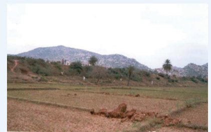
A weak tank bund
