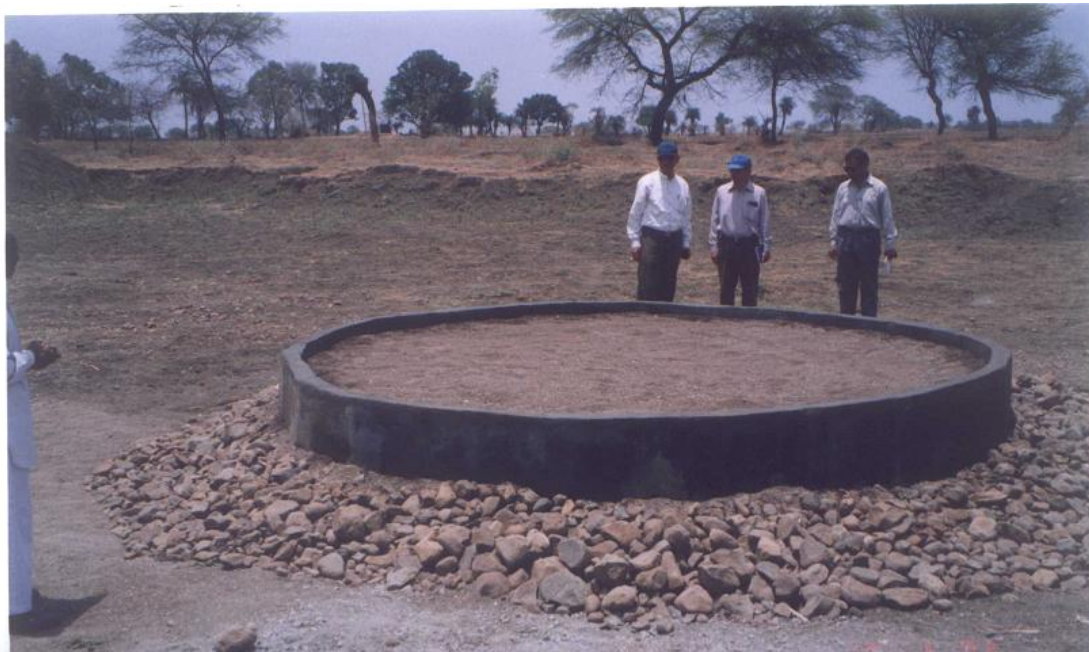
Fig. 8 - Percolation Tank with Recharge Shaft at Randan Khedi, District, Dewas, M.P.
