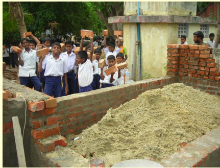
School children of P.R. Puram actively participated while constructing of toilet at the school
