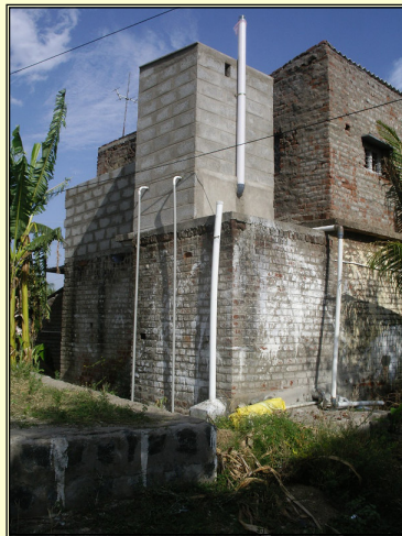
A view of the HCEST with separate pipe line for mud pot and filter bed.
