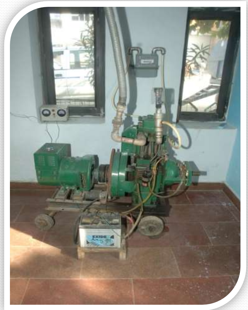
Biogas used for electricity generation
