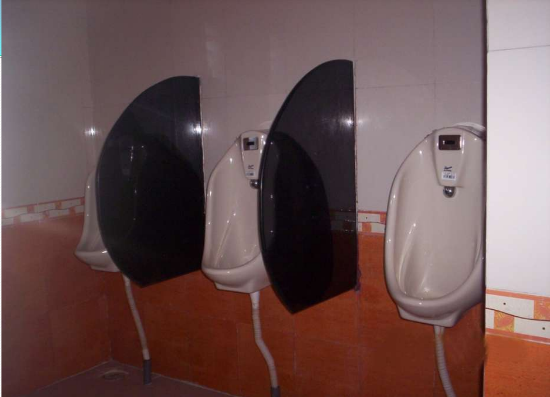
Urinals installed with sensor system
