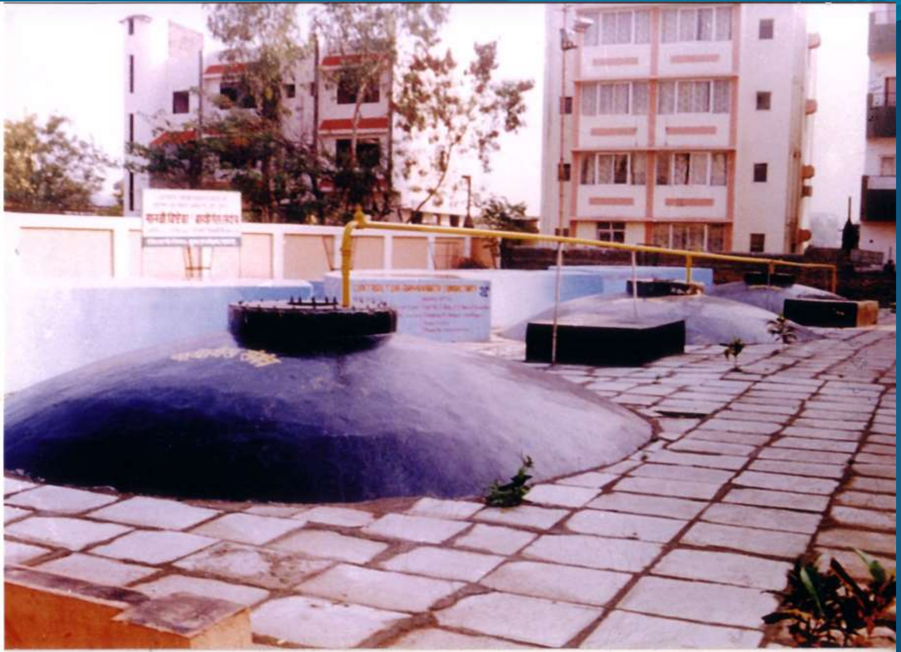
Biogas generation at Sulabh Toilet Complex, Shirdi, Nasik, Maharashtra
