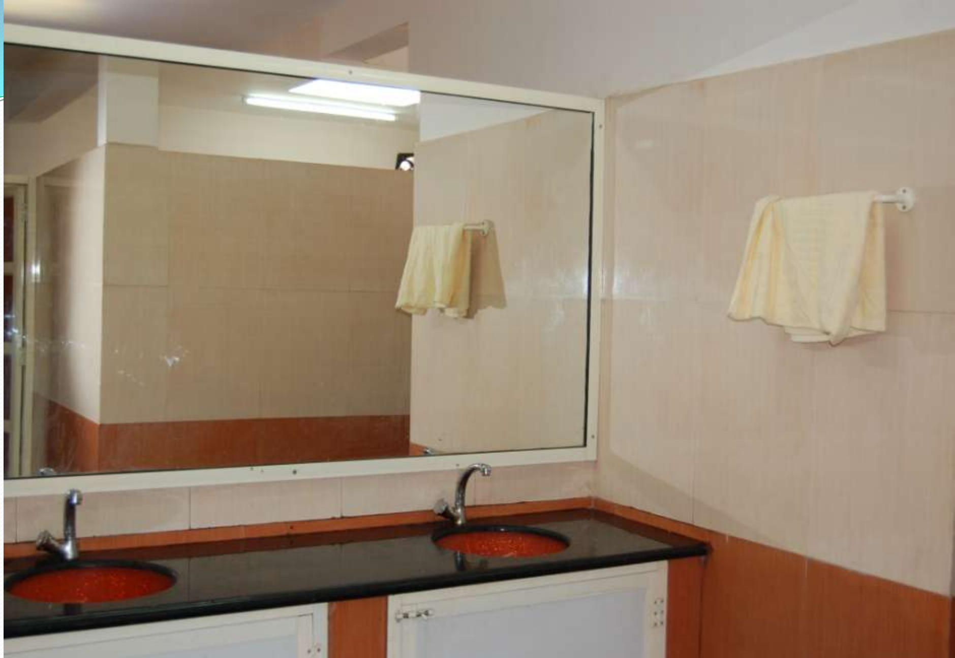
Water Tap fitted with Sensors
