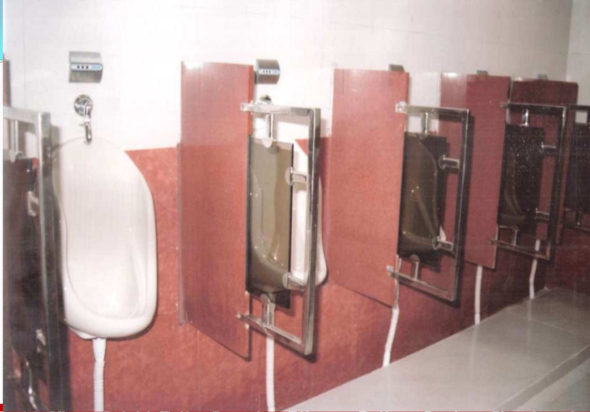
Inside View - Sulabh Toilet Complex, Bilaspur Railway Station, Chattisgarh
