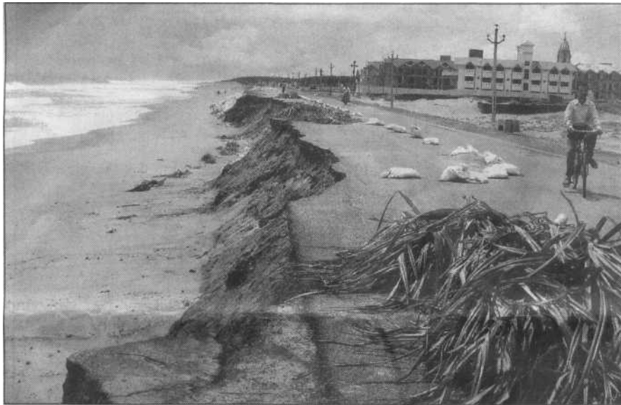
A part of seaside ring road in Orissa's temple town of Puri which has been washed away by menacing sea waves.
